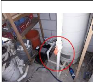
Main Water Valve: In the shed
