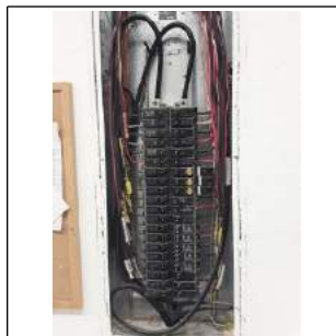
The breakers are in good physical condition
