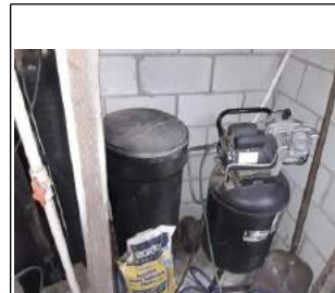
The water softener is in good working condition
