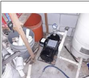
Well pump is new
